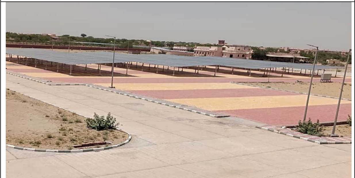
Photo 7.6: Solar power plant of 500KW capacity installed in the campus for generating clean energy for the campus and also providing space for vehicle parking
